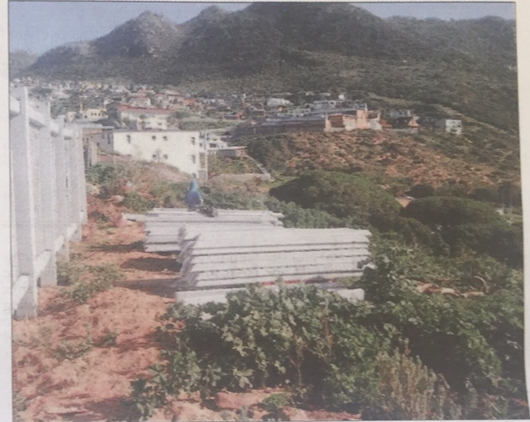
■ City officials are busy erecting a fence on Erf 8474 known to locals as the
